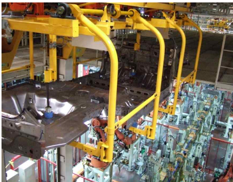
Overhead Electric Monorail System PROTON Body Shop Under Body
